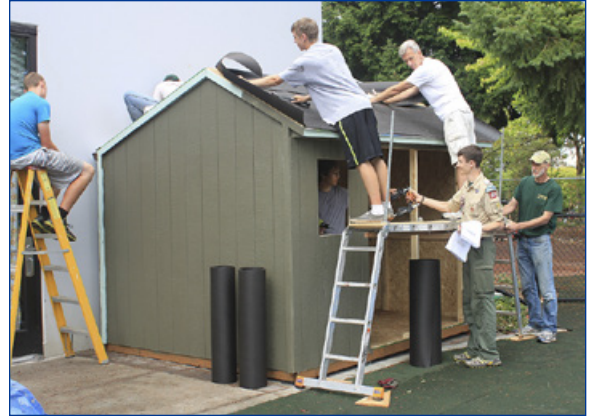
Tar-papering the shed roof are Troop 618 members Bobby Hagerup of Cedar Mill and Ed Herinckx, standing on scaffold. Logan Keith (in window) accepts wood clamps from Matthias Guenther. His father, Mark Guenther, is at right. On the ladder is Glenn Miller. Atop the roof, facing away, is Assistant Scoutmaster Eric Delaney of Cedar Mill.
